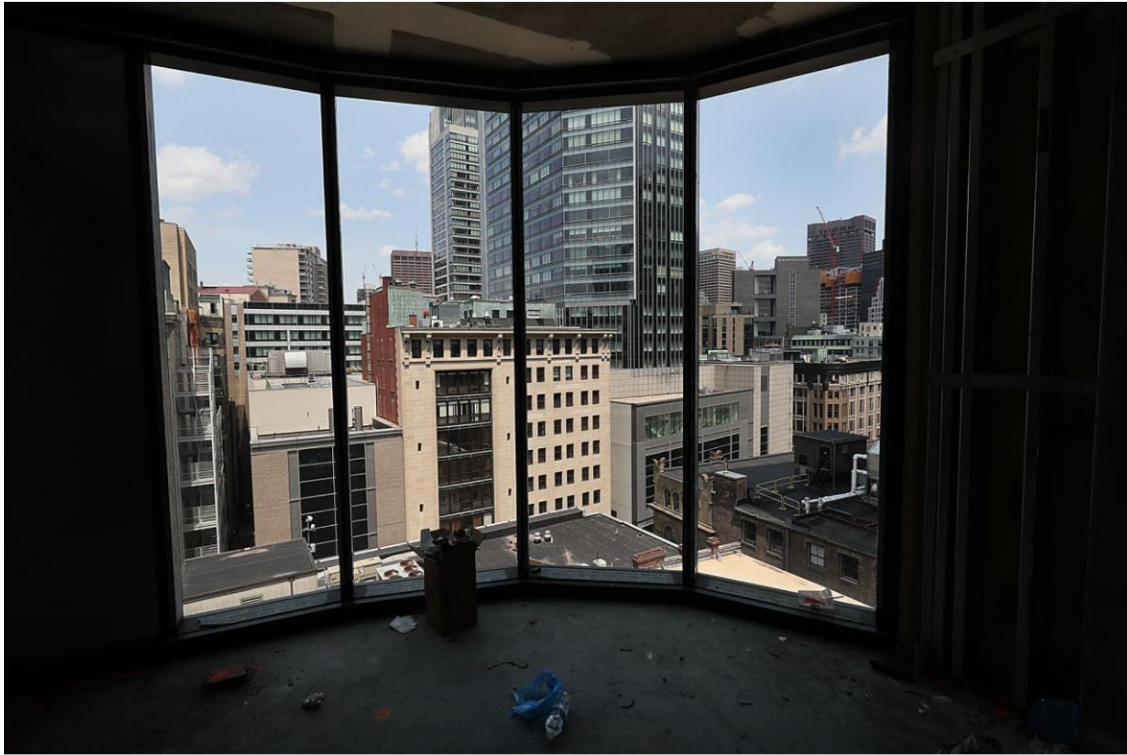
A unit under construction in The Parker condo building. SUZANNE KREITER/GLOBE STAFF
