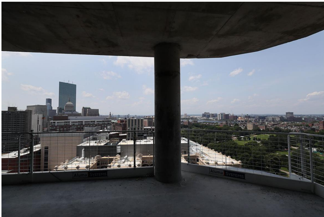
A condo unit under construction in The Parker on Lagrange Street in Boston. SUZANNE KREITER/GLOBE STAFF
