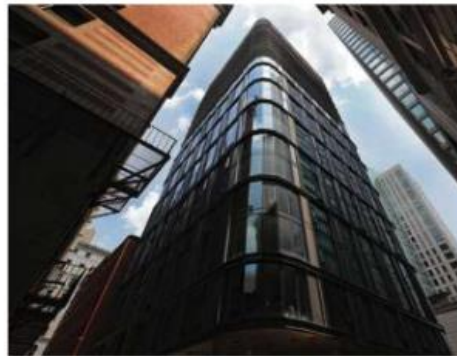
Top, a unit under construction at The Parker (above), a luxury condo building on Lagrange Street with units overlooking Boston Common.
